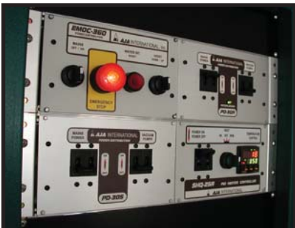
POWER DISTRIBUTION MODULES
